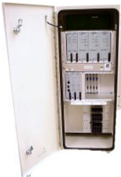
Figure 20 Field Shelf Enclosure
